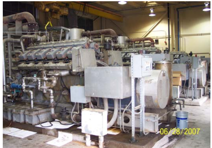
Figure 1. V-12 engine/generator sets.
