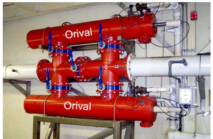
Figure 2. Filtration system: Two Orival OR-12-PS filters with manifold.
